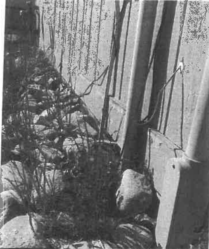
Bottom siding/board in poor condition and needs replacement:
